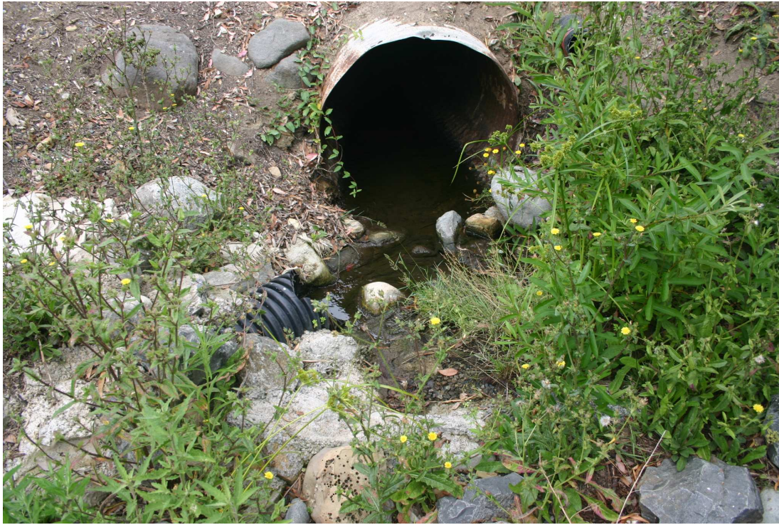
PHOTOGRAPH 1: View of 36-inch pipe discharging to 12-inch pipe at northern end of relict drainage feature.
